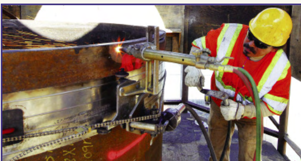
Luis Garcia, from Los Angeles, fresh-heading top of pile to permit attachment of the next section.
