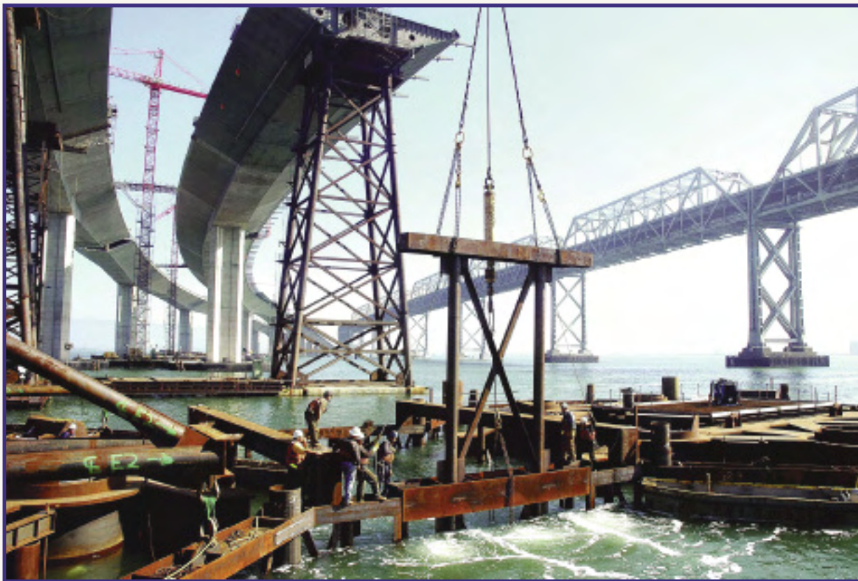
Local 34 crew installs last section of template to guide piles at T-1 site.
