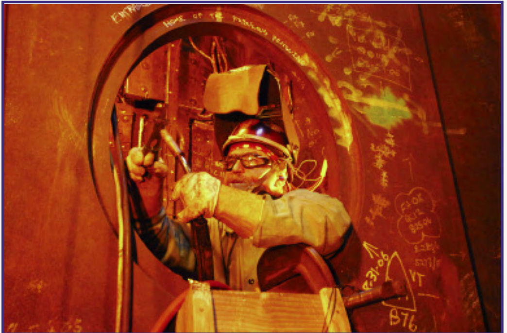
The hottest job on the bridge—Randolph Dolan, in protective clothing inside steel footing, welding connector plate to pile. Plates were often heated as high as 275°F.
