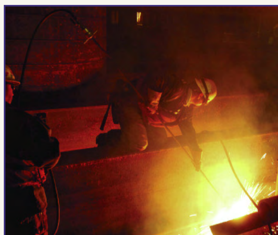
Doug Ailes cutting off the falsework, which held up piers that supported the bridge.
