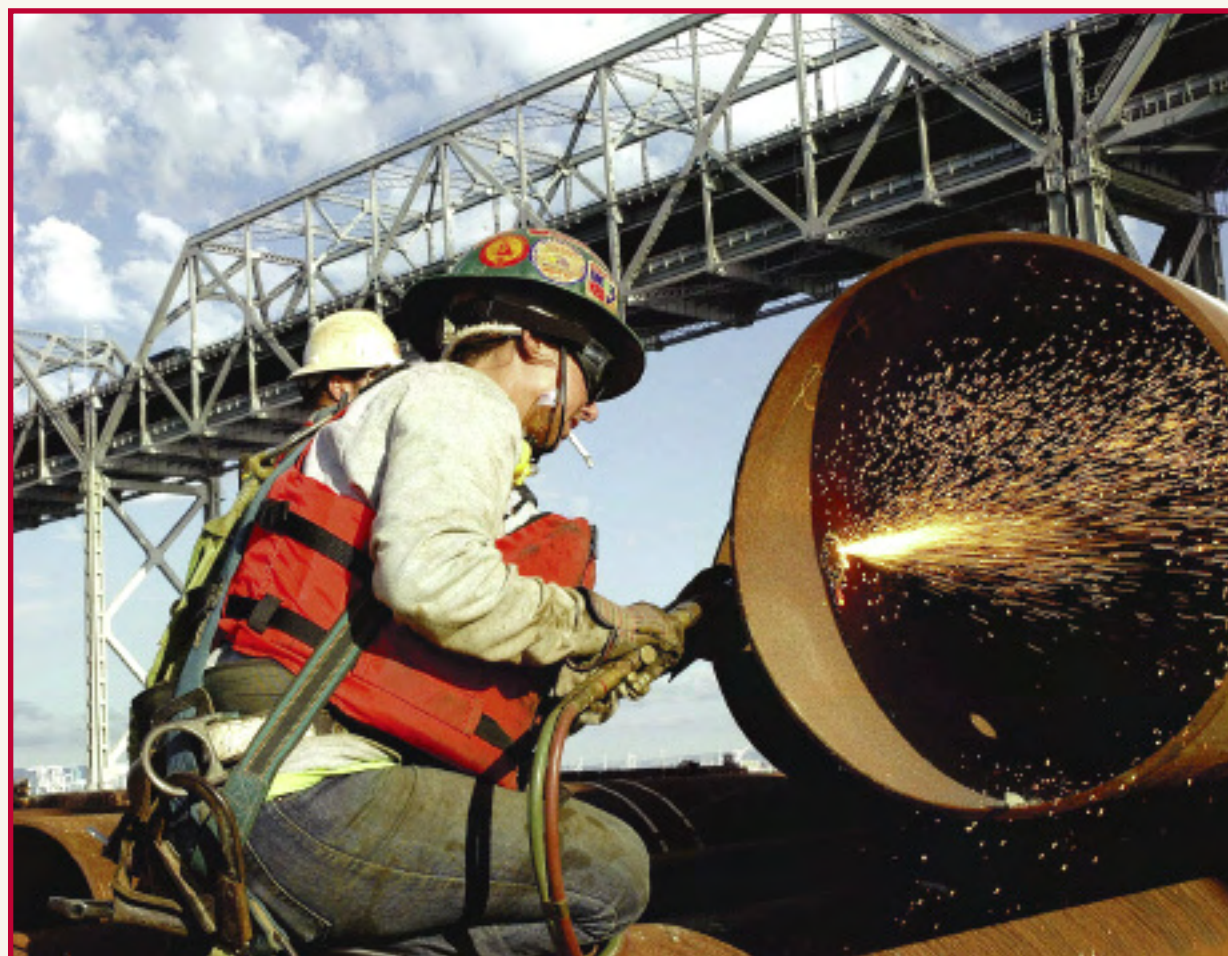
Cory Pakes, apprentice of the year in 2005, burning holes in the panels that will hold up the templates, which control piles for the new east span.
