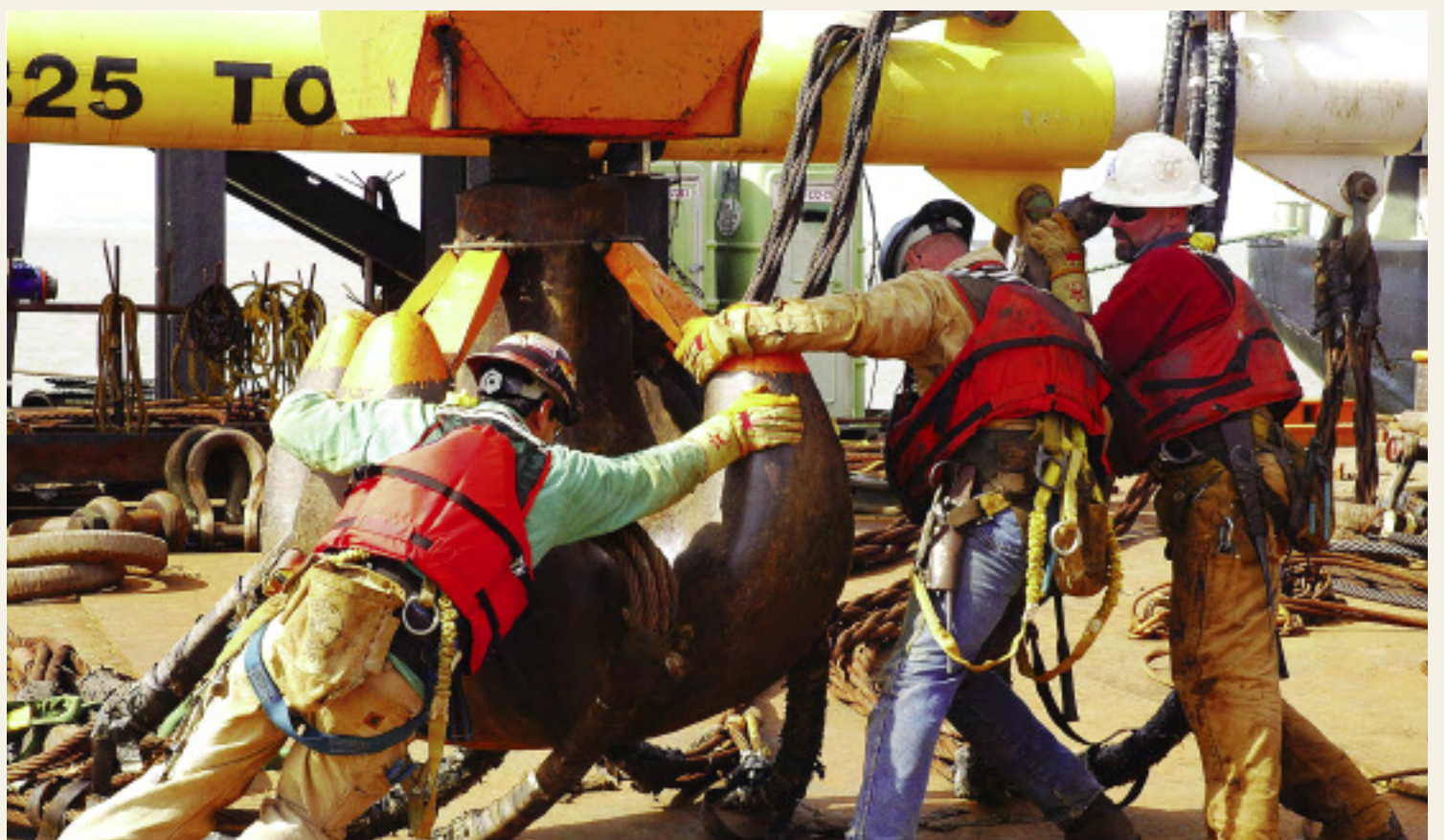
Doug Ailes and Dave Lang rig the crane to lift a 325-ton spreader bar.
